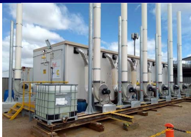
Figure 2 : FYI's pilot plant
